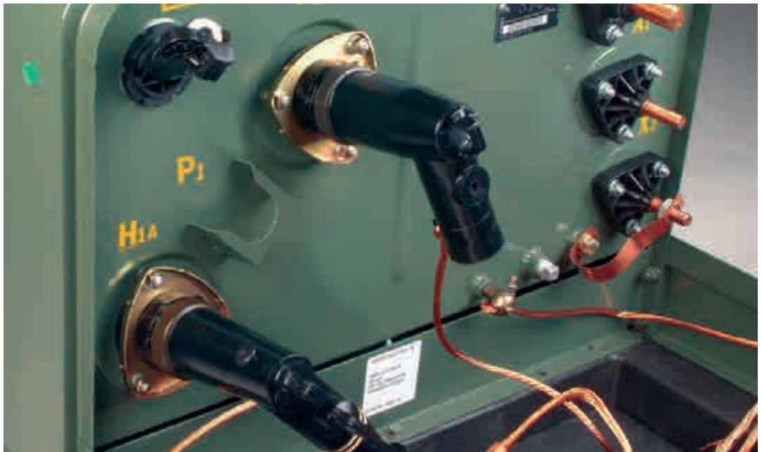
Two-bushing transformer To add surge protection to a two-bushing transformer at the end point of a radial-feed circuit, add an elbow arrester to the unoccupied bushing or use a bushing arrester.
